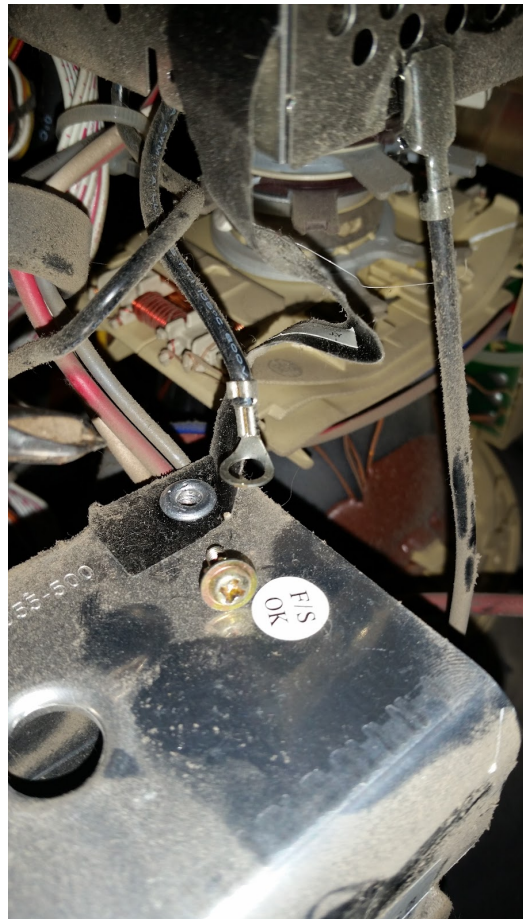
Grounding wires detached to get to circuit board
