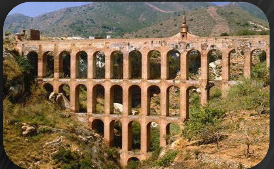
Figure 6: Vibration-based and neural network tests are conducted to assess the structural integrity of various components of the aqueduct.
