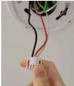
The smoke detector is connected by a 3-way switch to the house, which has a red, white, and black wire.
